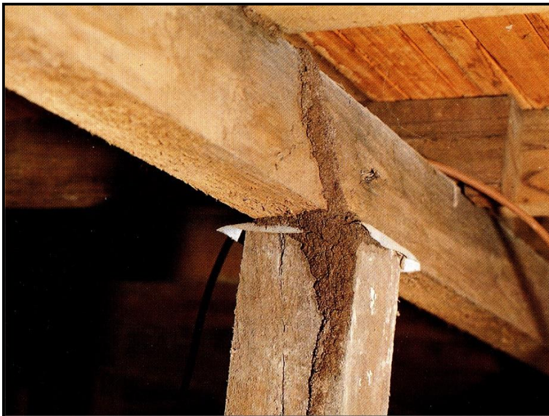
Termite mud tube on wood support structure
